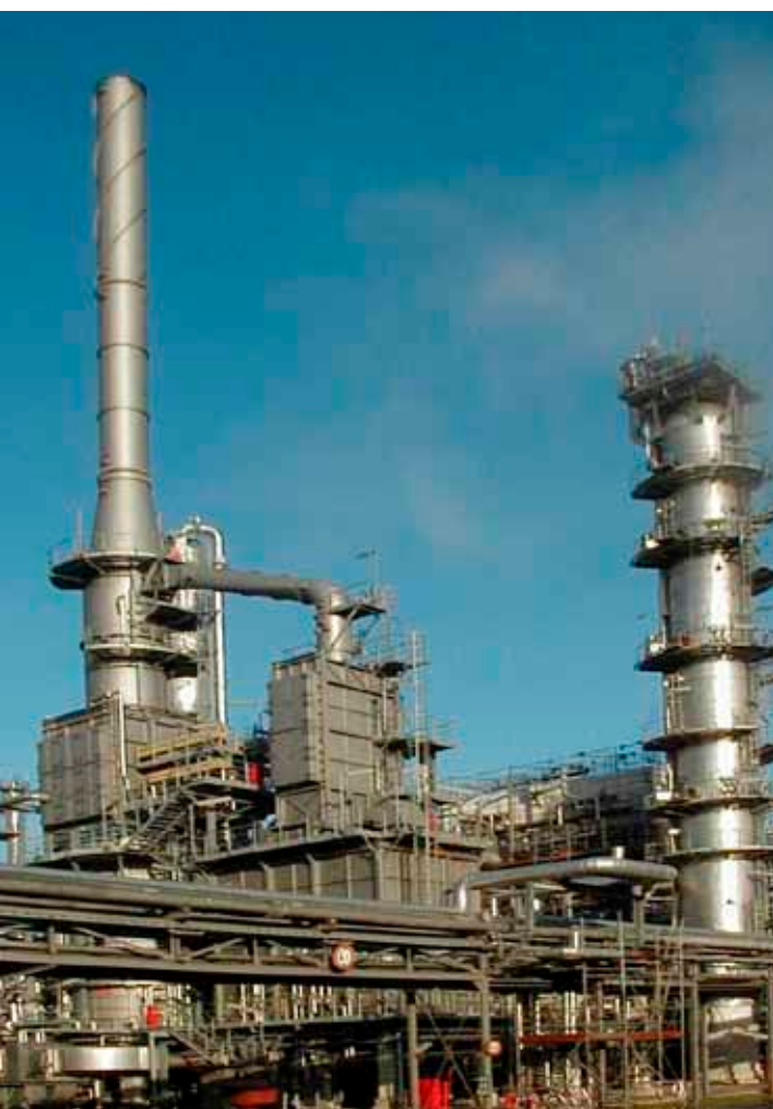
Hydrocracker in Heide
