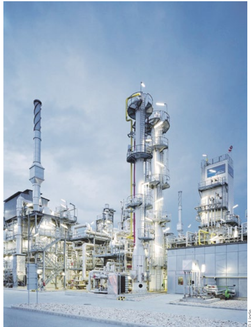
HyCO-Steamreformer-Anlage in Kazincbarcika, Ungarn.
