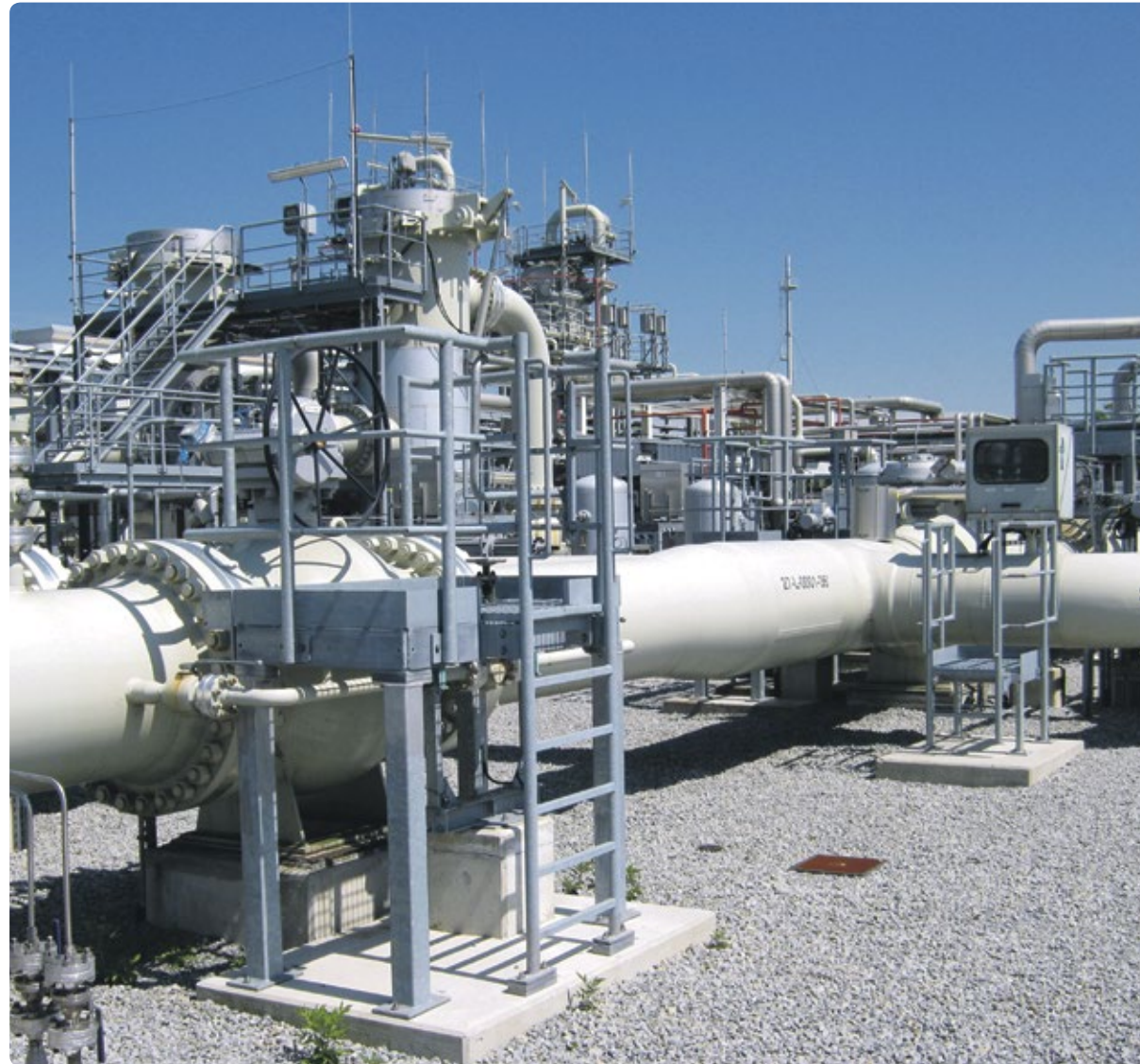
Abb. 1: Erdgasspeicher Etzel Gas-Lager in Ostfriesland.
