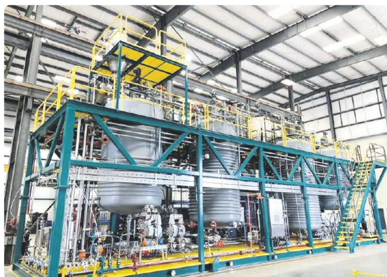
Green Li-ion's modular units are customizable to fit any battery cell producer's needs and deploy quickly into existing facilities. The plant at Atoka, OK, US, is the first producing pCAM from black mass in North America.
