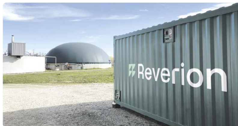
Reverion's micro power plants enable a highly flexible and efficient decentralized energy supply.
