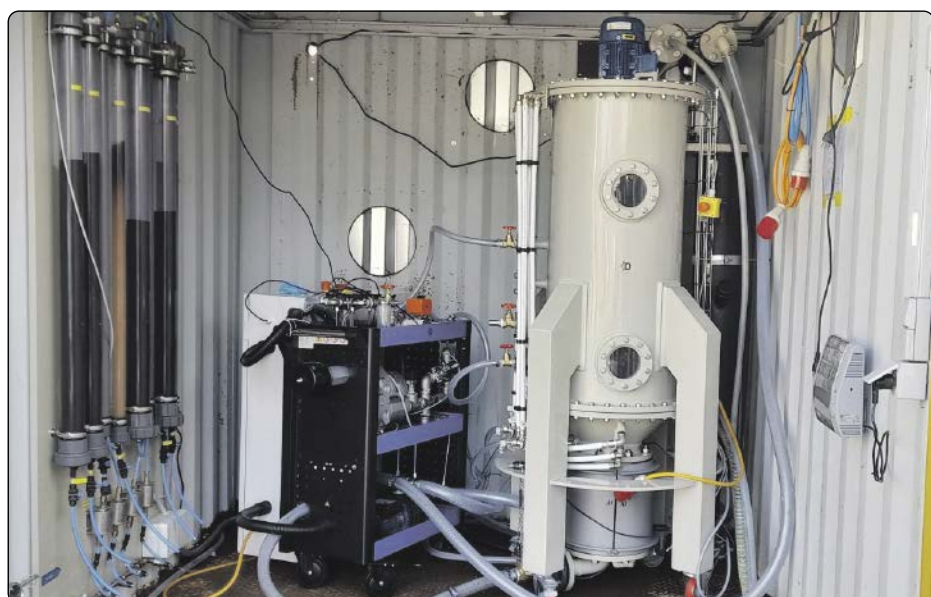
Oxyle's wastewater treatment platform (shown is one of the pilot units) includes modular reactors, nanoporous catalysts, and real-time monitoring services powered by clean energy sources.
