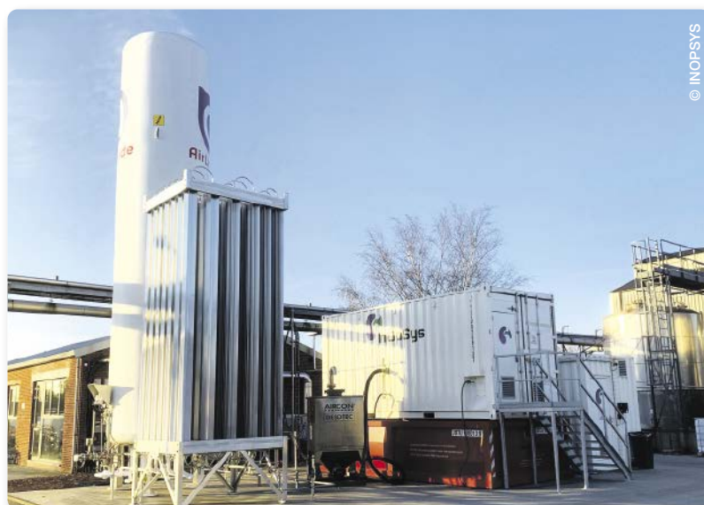
One of the running on-site installations recovers valuable palladium, used as a homogeneous catalyst by the customer, and purifies the wastewater, closing the loops.
