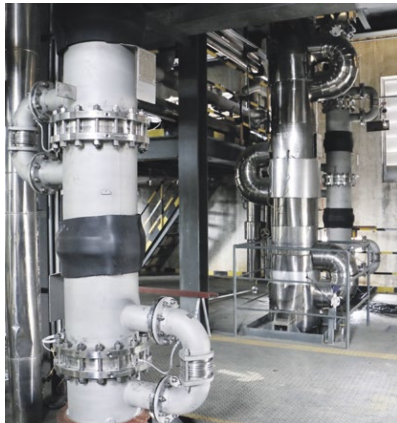
Integration of the continuously running Miprowa flow reactors into the existing building infrastructure at Shaoxing Eastlake in China.
