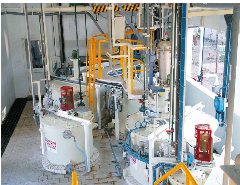
Fentox pretreatment of toxic wastewater from production of crop protection agent
