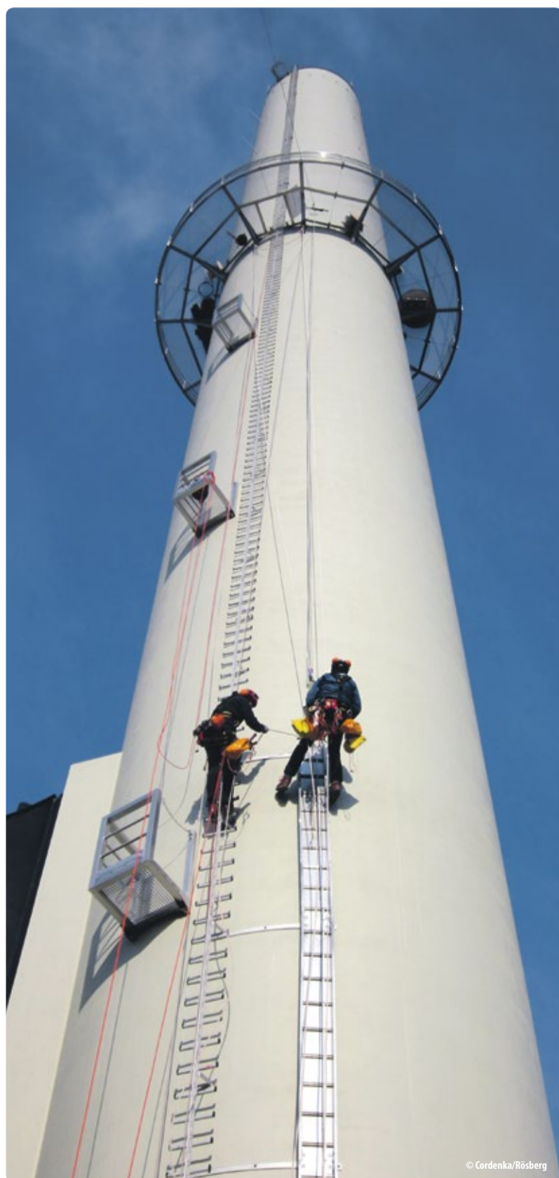
The new exhaust air extraction system: one of the two new exhaust chimneys with emission measuring points on the 43-meter-high working platform.
