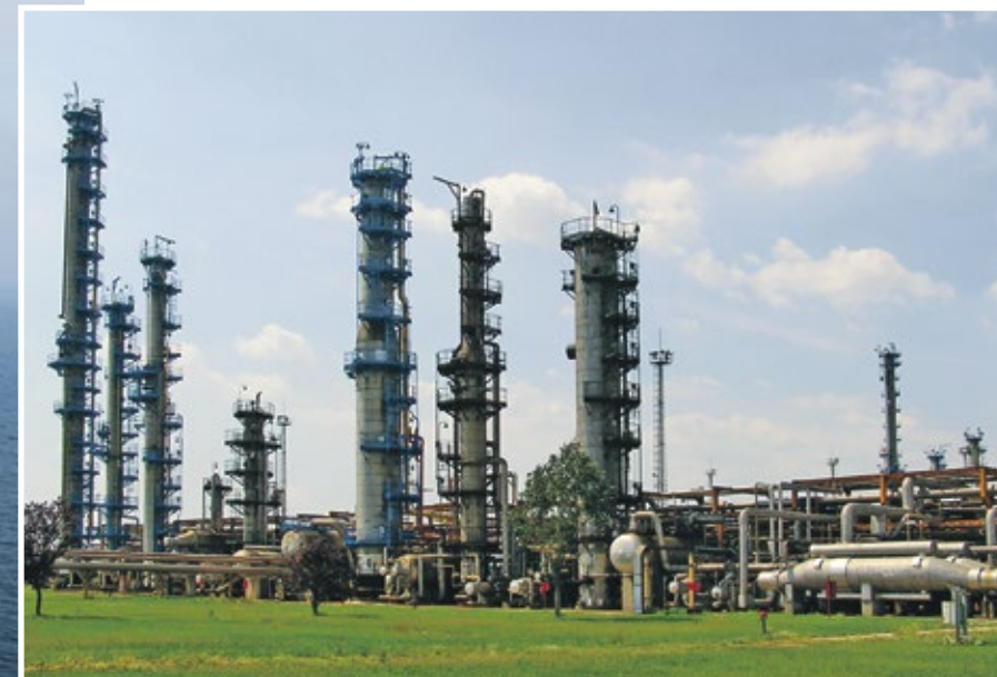
Emerson's SmartProcess Distillation Optimizer has been applied to five of the six gas distillation columns at MOL's Algyő gas plant in Hungary.
