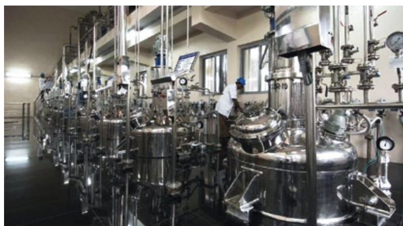
Dr. Reddy's Active Pharmaceutical Ingredients Unit Bollaram, Hyderabad, India is one of many state-of-the-art production facilities for APIs in Asia.
