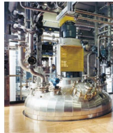
Glasslined apparatus in active ingredient production
