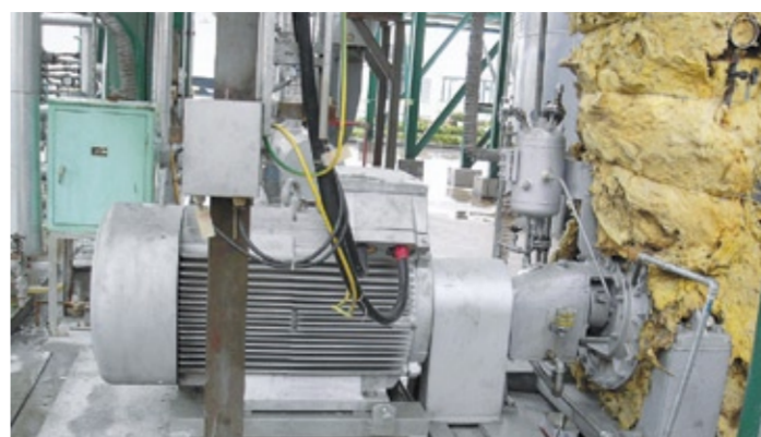
Pump installed in a plant
