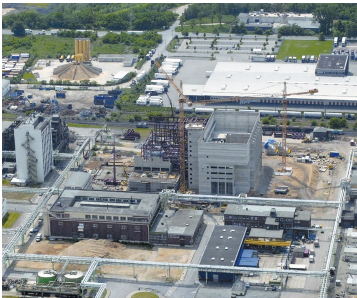
Site Knapsack overview in June 2007, on the right the new power plant of Statkraft, in front the plant of Sotec and InfraServ Knapsack under construction.
