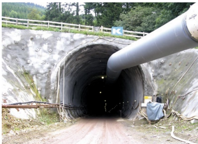
About 900 m stretch of pumping in the Blessberg Tunnel in Austria: Chains of pumps of such lengths and more are possible when connecting pumps in series
