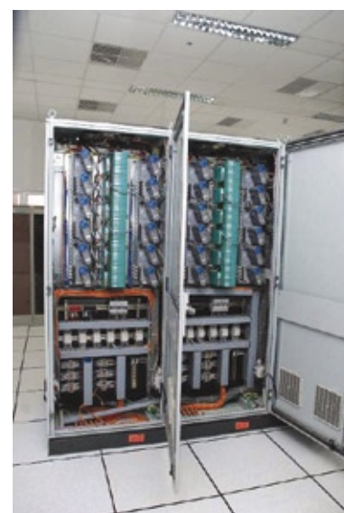
Fig. 3: Fieldbus power hub cabinets
