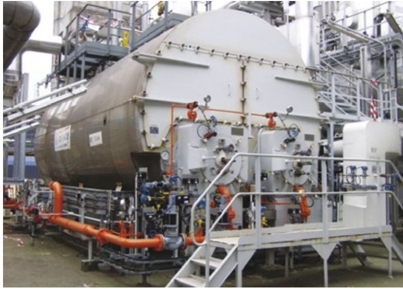
Total Petrochemicals Antwerpen meets operational, financial and environmental goals with boiler re-vamp project and advanced control solutions from Honeywell.
