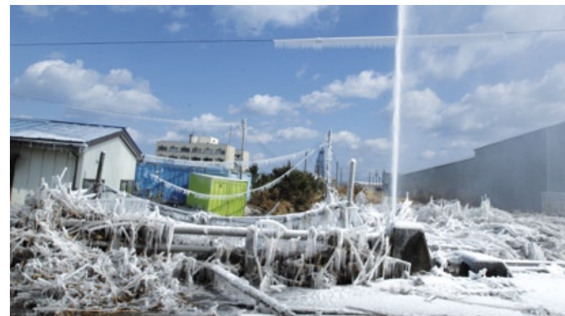
Damaged water pipe shoots water following earthquake off Japan's coast. (U.S. Navy photo by Chief Mass Communication Specialist Daniel Sanford)
